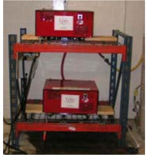
Custom Installation 2 Alkota All Electric Power Washers on a Custom Built Stand
